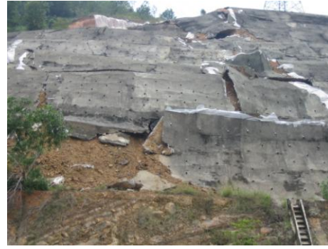
Figure 5. Photo showing the shortcrete failure area in slope while waiting to collapse in any time alone because of failure design and less monitoring (10th October 2006).
