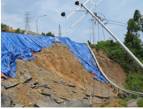
Figure 4. Photo showing the landslide embankment area has destroyed almost half road in Karambunai Resort junction area which collapsed in 10th October 2006.
