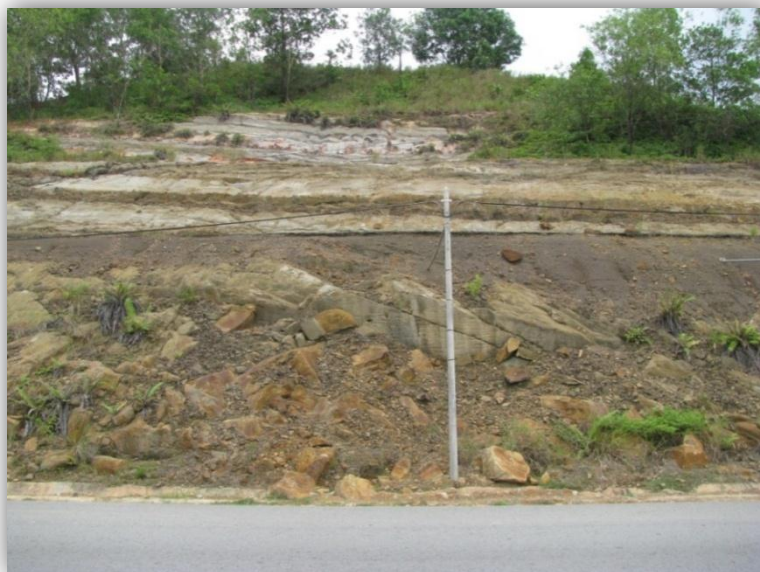
Figure 1. More than a cubic meter (m 3 ) fallen rock block at the bottom of cut rock at Slope 5.
